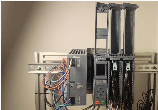
(a) PLC S7-1500
